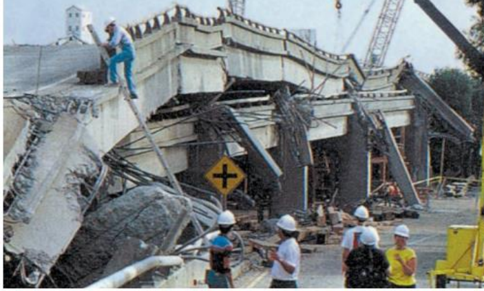
Figure 11.17 A part of the Cypress Freeway in Oakland California that collapsed during the 1989 Loma Prieta earthquake. [from: http://upload.wikimedia.org/wikipedia/commons/9/91/Cypress_collapsed.jpg ]
